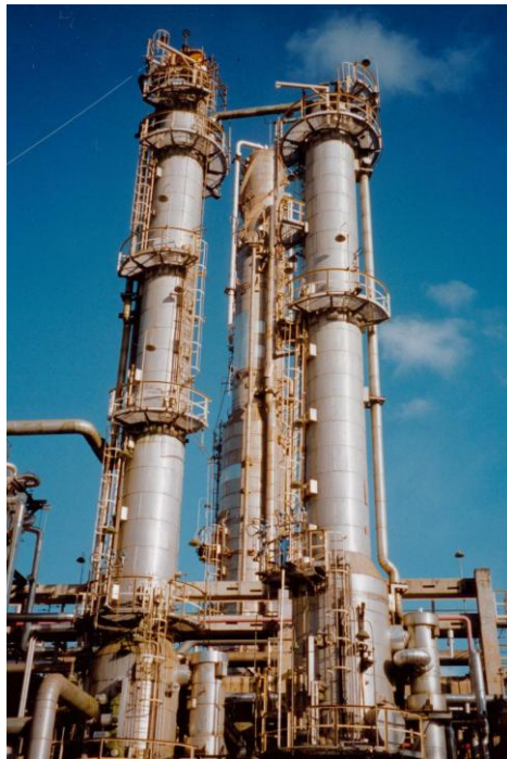
Figure 2. A typical industrial distillation column.
